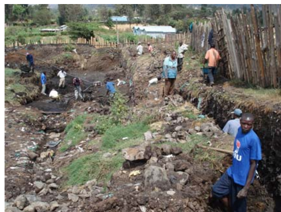
Work on the filtration ponds which must be finished by 20 th September 2008.
